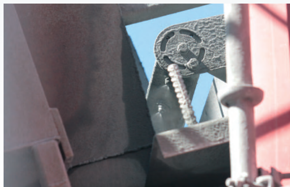
HA series misting nozzles at a conveyor transfer point
